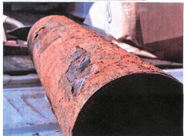
Section of Sherrard Street pipe taken out of service on December 14, 2009
