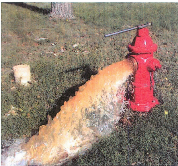
Typical flushing of Sherrard Street line.
