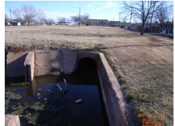
Looking east at the inlet headwall on the south end of the irrigation ditch.
