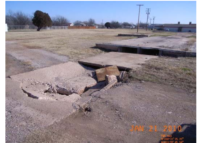
Collapsed box culverts north of Iowa Park Rd.
