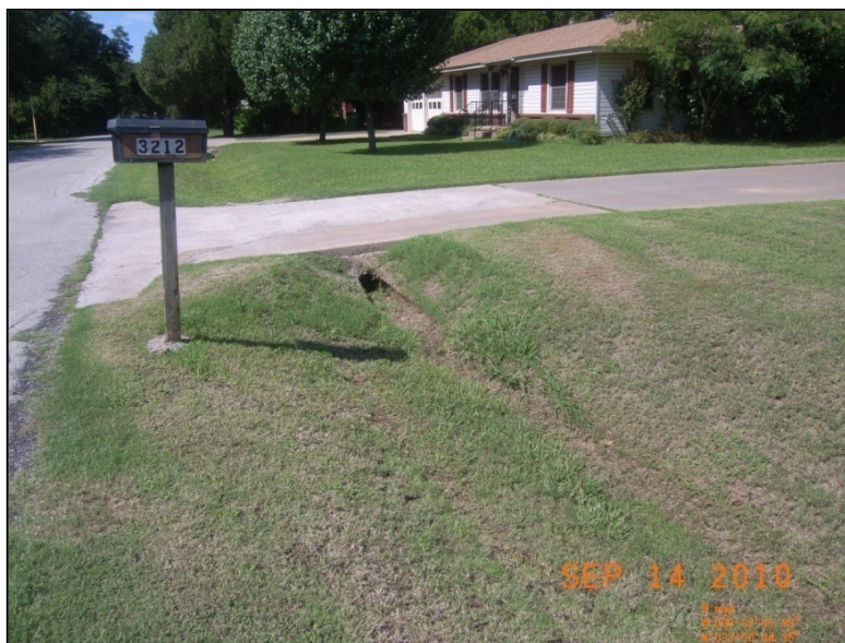
Photo 1 – A typical ditch and driveway culvert in the Wichita Gardens project area.
