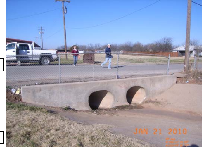
Outfall of East Plum Creek with 2-36" RCPs on the east side of Ridgeway Dr.
