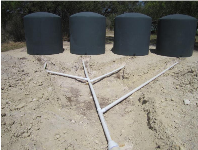
COLLECTION TANKS (3K GALLON) CONNECTED TO PLENUM
