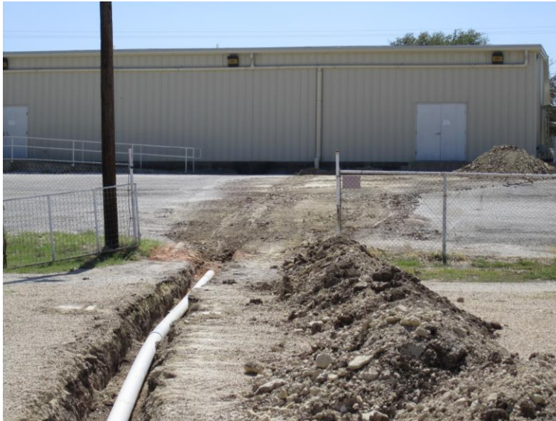
SIX INCH TRANSFER PIPE CONNECTING CIVIC CENTER WITH COLLECTION TANKS
