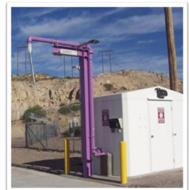
Figure 10: Reclaimed Water Dispensing Station (Source: El Paso Water Utilities)
