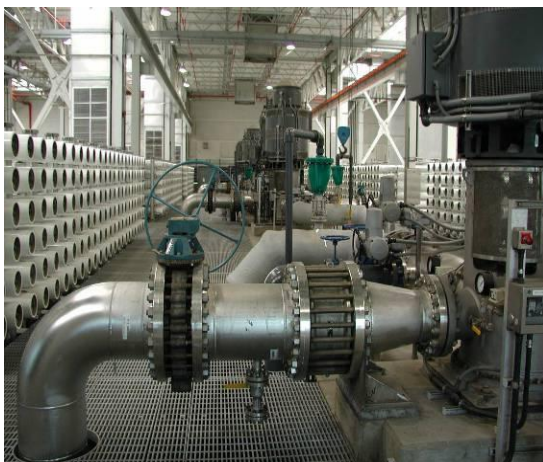
Figure 16: Orange County Water District, Groundwater Replenishment System Advanced Purification Facility, reverse osmosis units (Source: Dr. James Crook)
