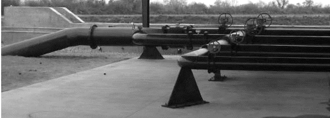
Closed pipe manifold.
