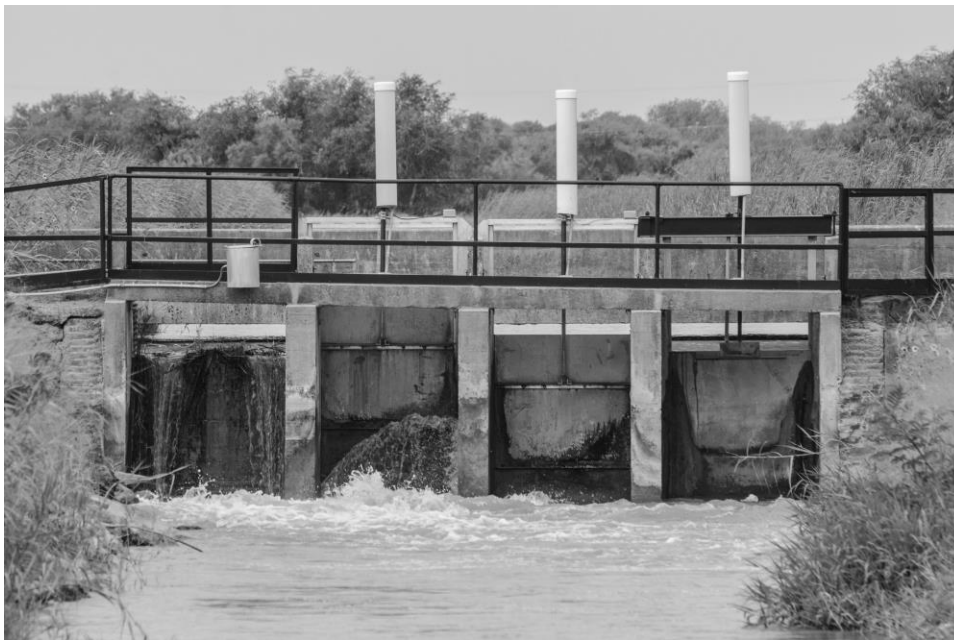
Automated gates in action.
