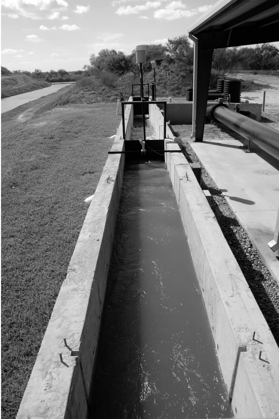
Flume with water showing auto-gate.
