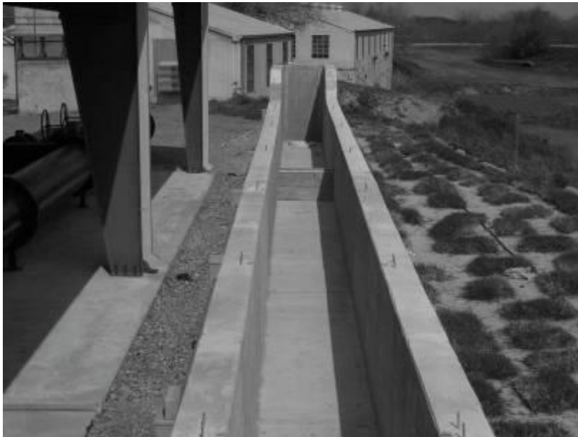
Flume inlet with sharp crested weir.
