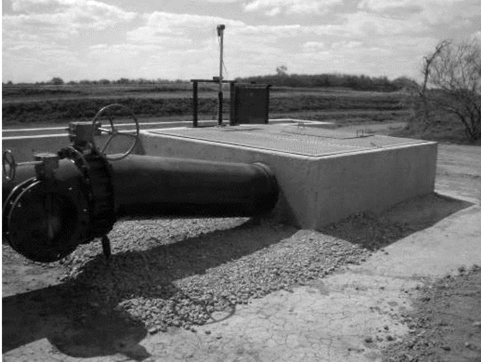
Manifold discharge and calibration tank.
