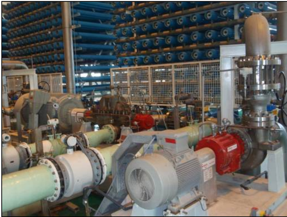
Figure 1 – High Pressure Pump, Circulation Pump and Membrane Array
