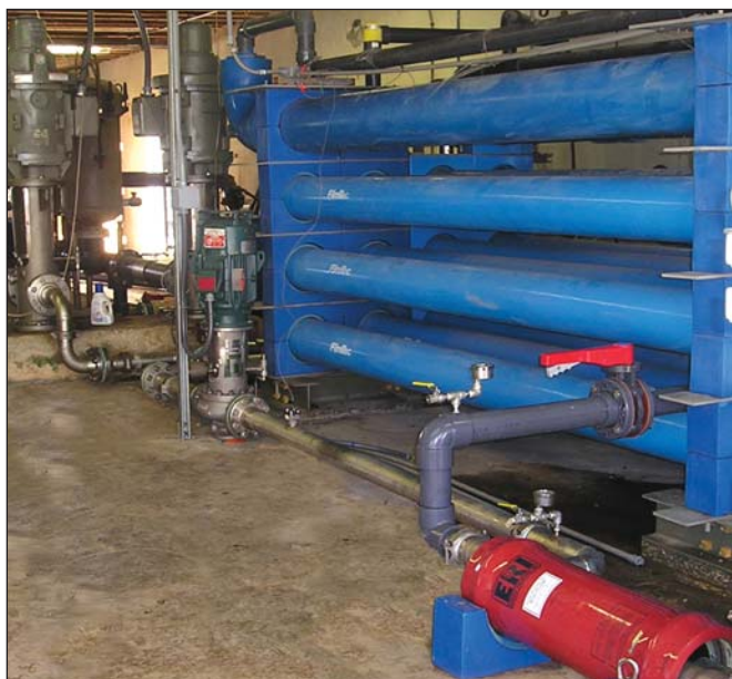
Energy Recovery Inc.'s retrofit installation at the Ocean Reef Club in Key Largo, Fla., shows (from left to right) the PX220-B, the reverse osmosis rack, the booster pump, and the high-pressure pumps.
