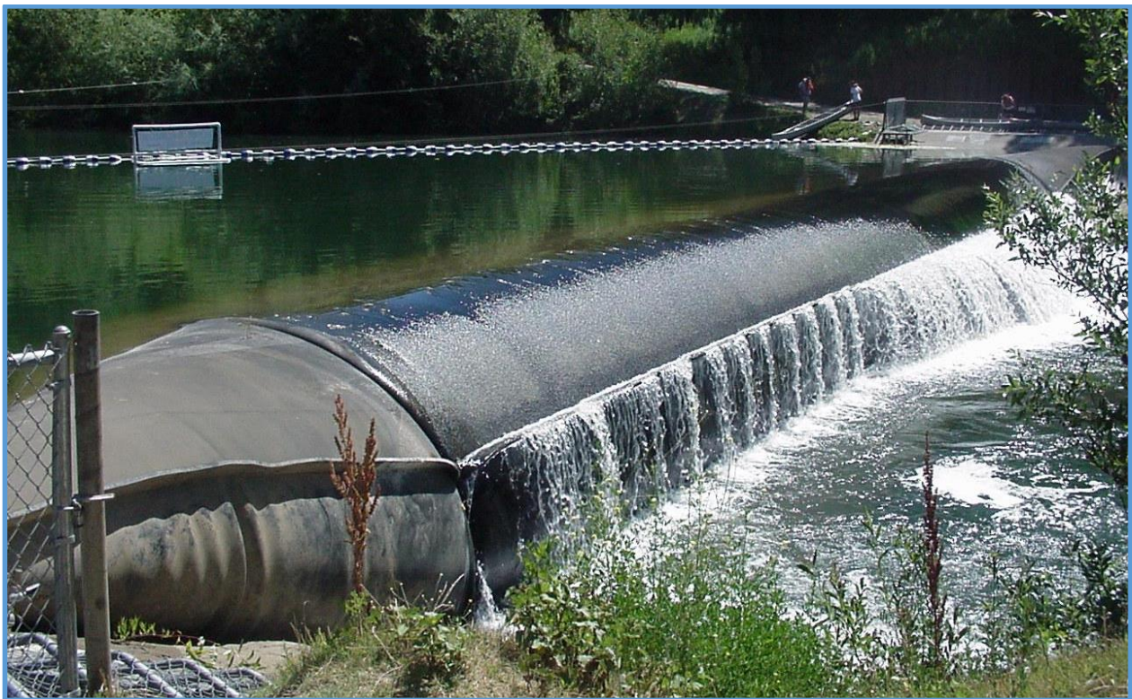
Figure 3.2.1-8 Inflatable bladder dam (Photo: http://ca.water.usgs.gov/user_projects/sonoma/sonomapics.html )
