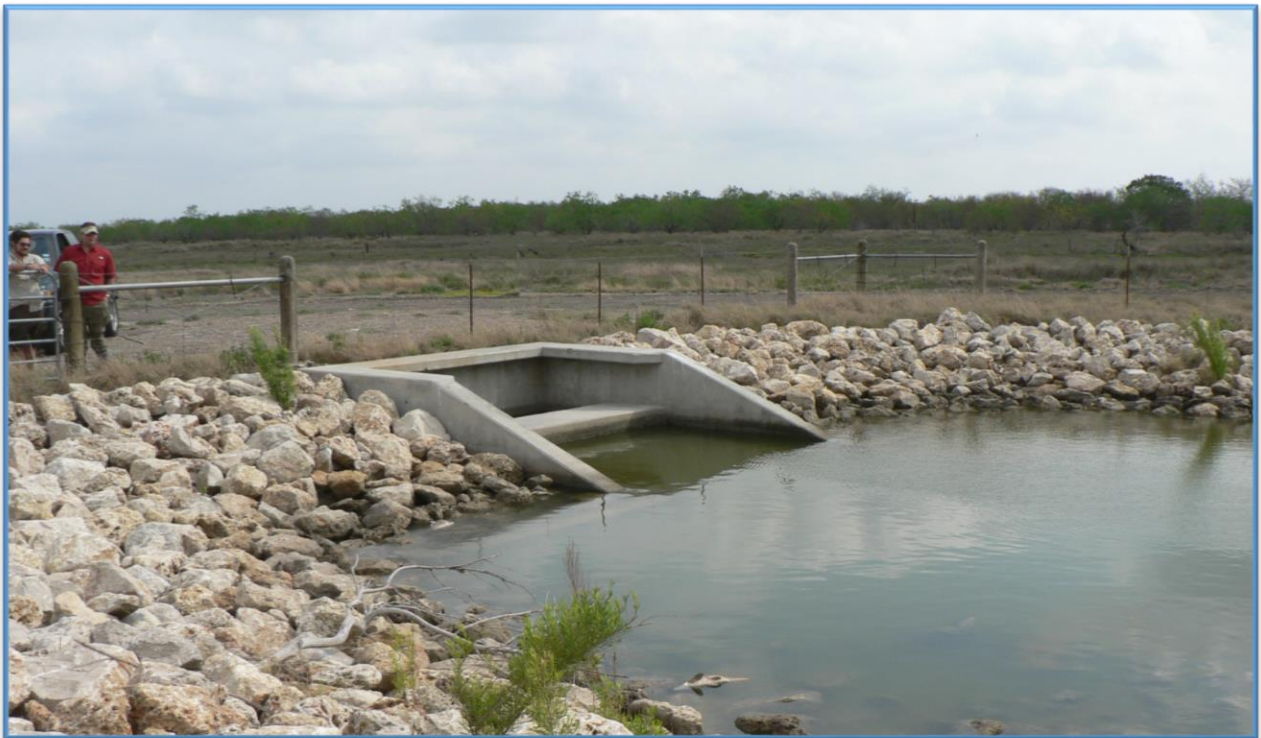
Figure 3.2.3.2 Concrete Outfall for City of Corpus Christi’s Freshwater Diversion Pipeline to Rincon Bayou
