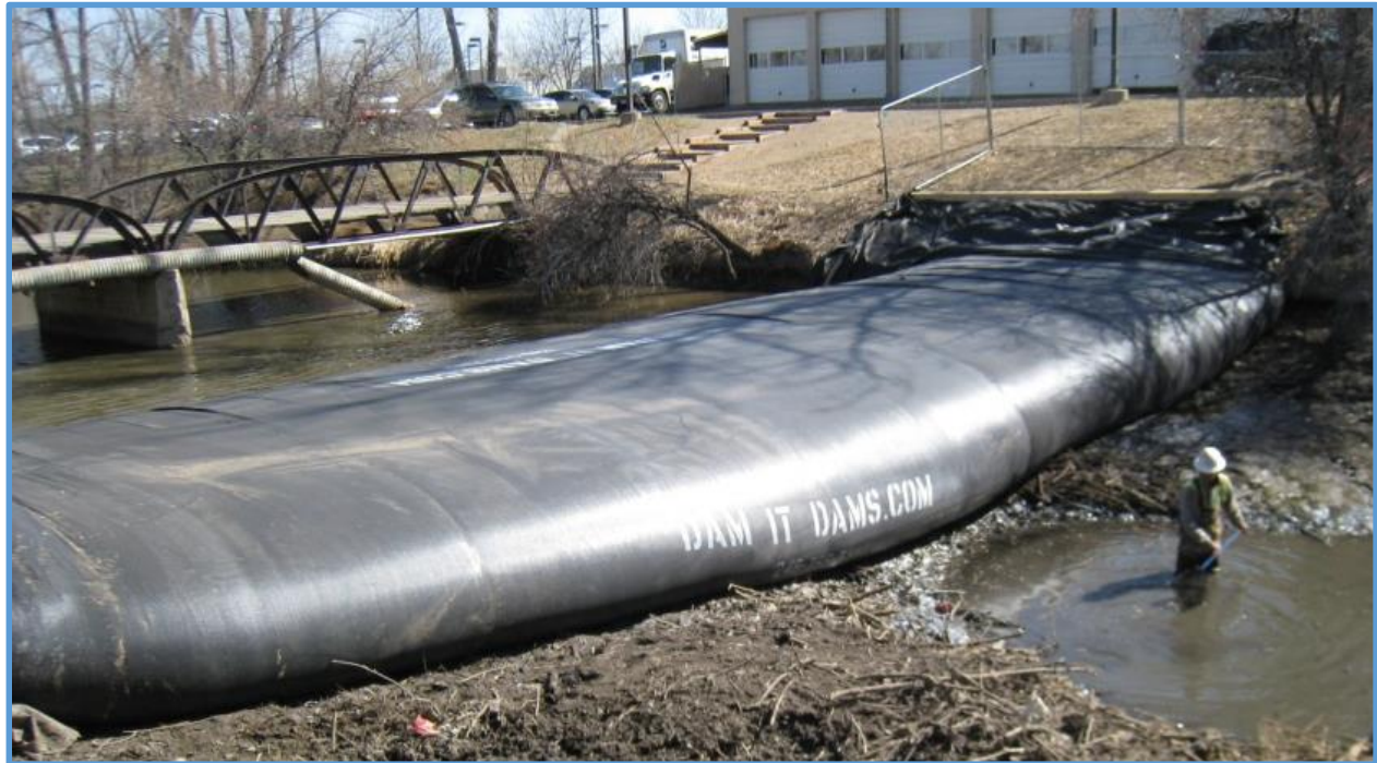
Figure 3.2.1-7 Water filled bladder dam (Photo: http://www.damitdams.com/images/portfolio/rivercrossing/IMG_4435.jpg )
