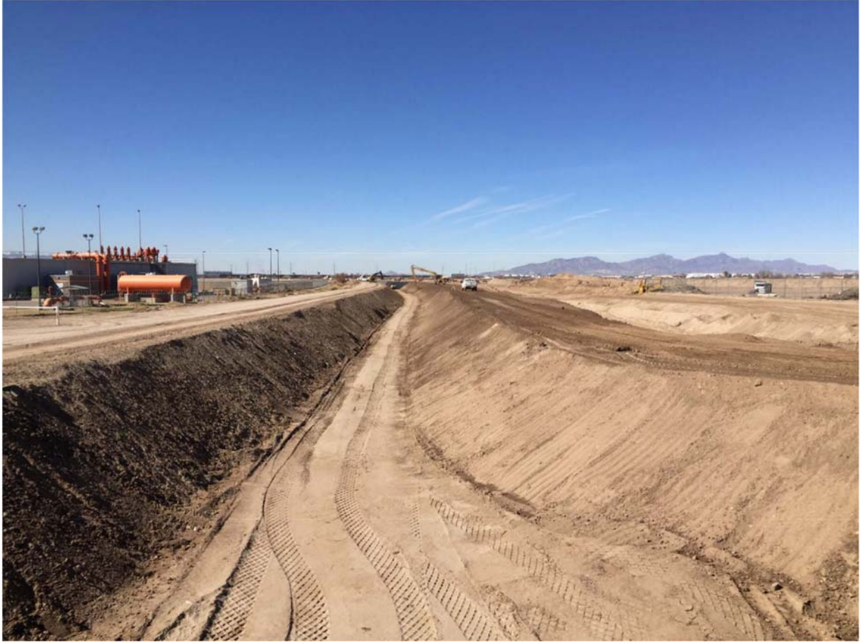
Location 6. Earthen cross sections and transition to the Pan-American Bridge were completed. Photo dated 2/4/16.
