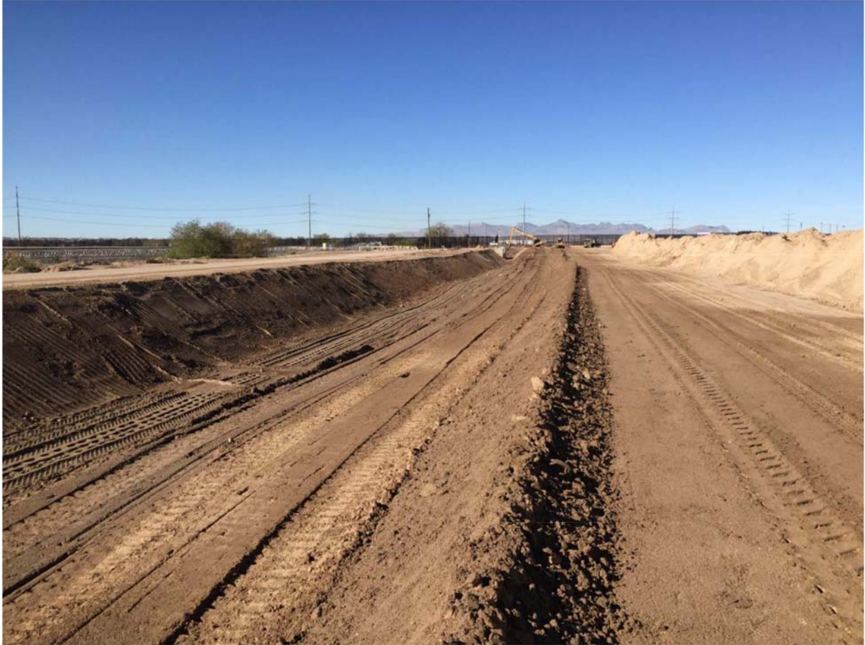
Location 5. Continued earthwork and canal shaping at Location 5. Dirt piled on the right canal bank was used to narrow the canal cross-section. Photo dated 11/18/15.
