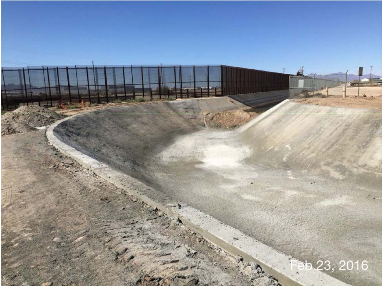
Location 1A. Transition from the American Canal to the Riverside Canal has been completed. The canal is fully lined. Photo dated 2/23/16.
