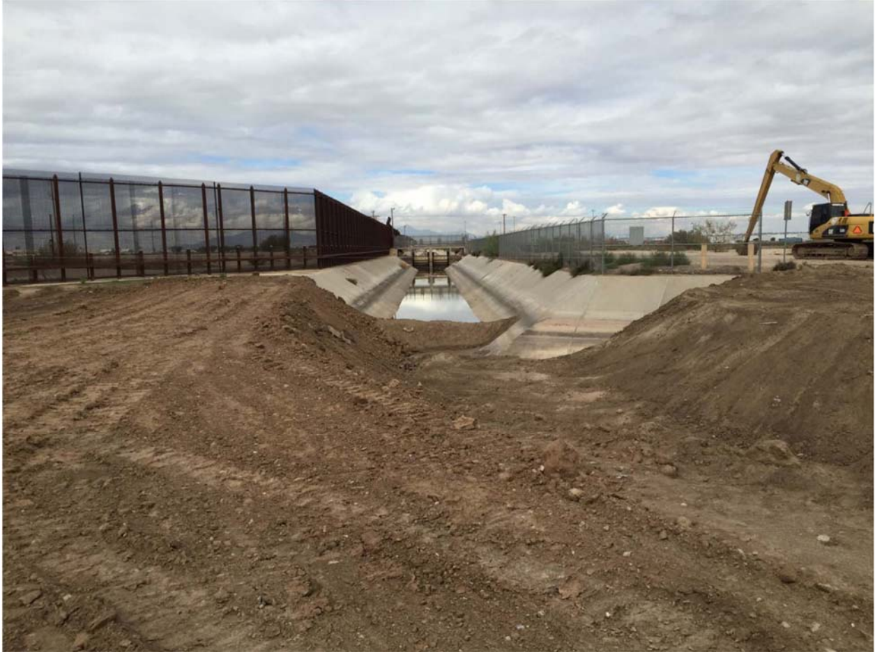
Location 1B. Initial earthwork at the Riverside Canal heading. An embankment was made to stop stormwater flows at the American Canal during construction. Photo dated 10/30/15.
