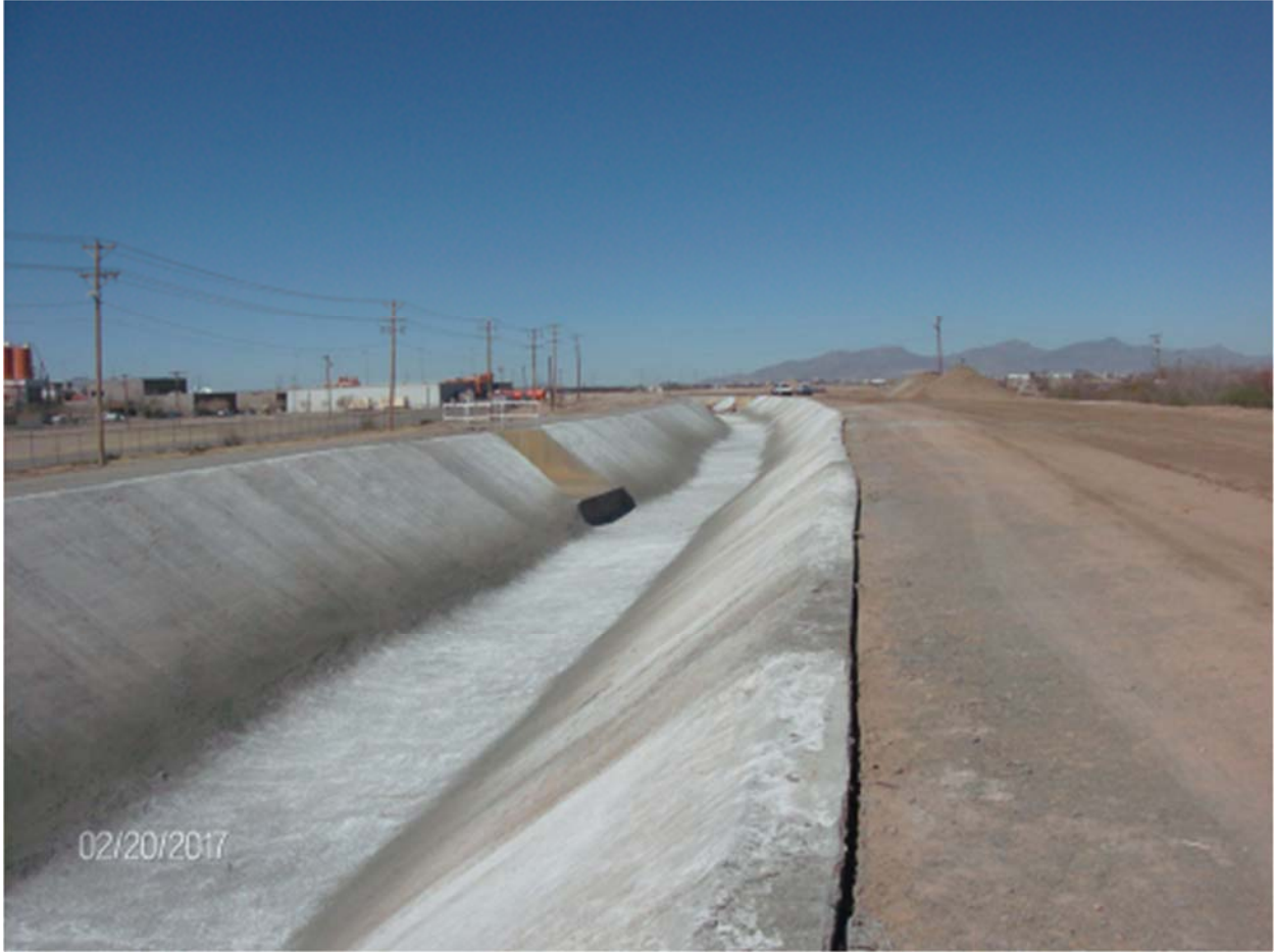
Concrete lining completed downstream from the treated wastewater discharge structure from the Robert Bustamante Wastewater Treatment Plant. Photo dated 2/20/17.
