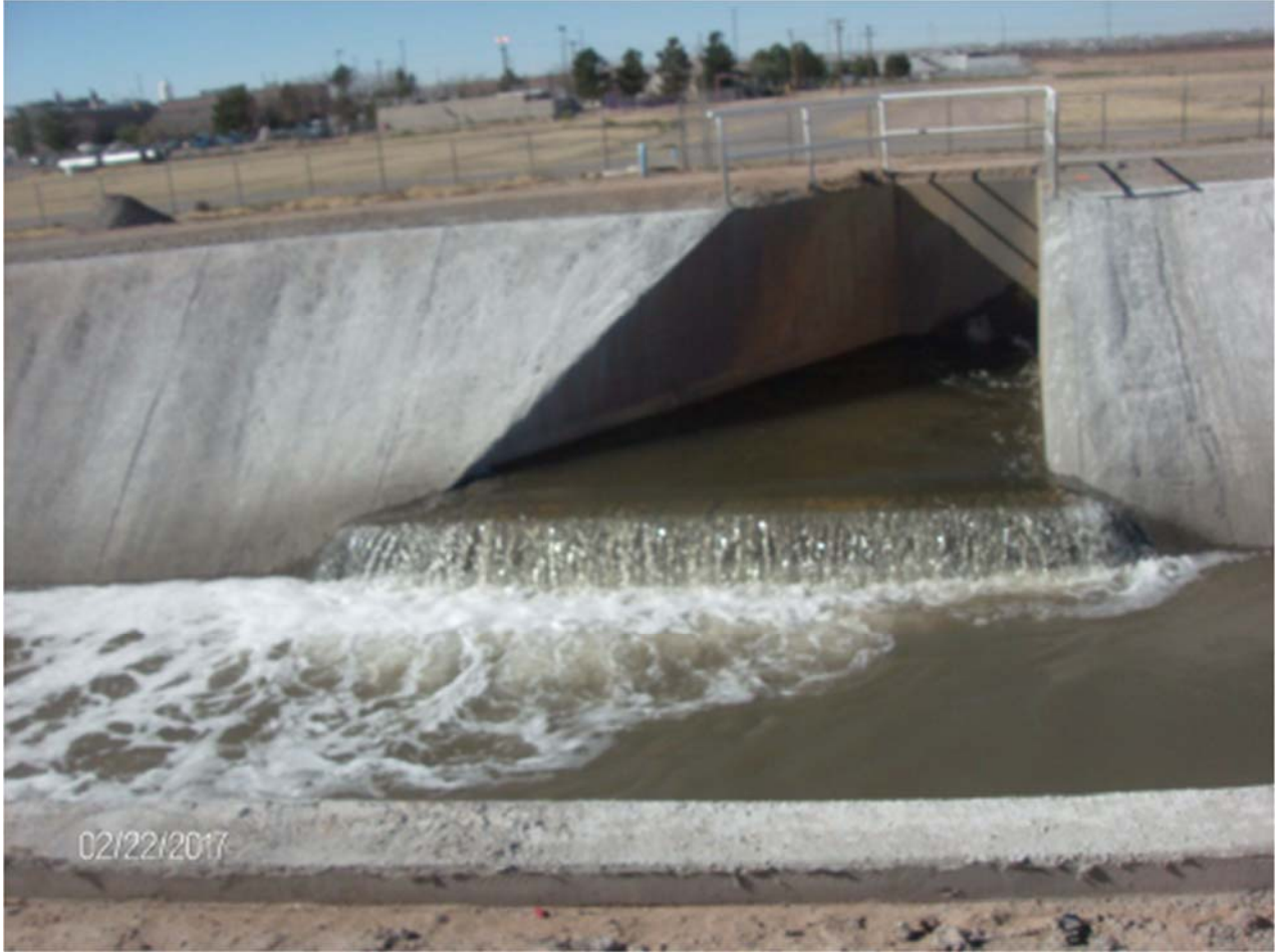
Discharge structure from the Robert Bustamante Wastewater Treatment Plant. Photo dated 2/22/2017.
