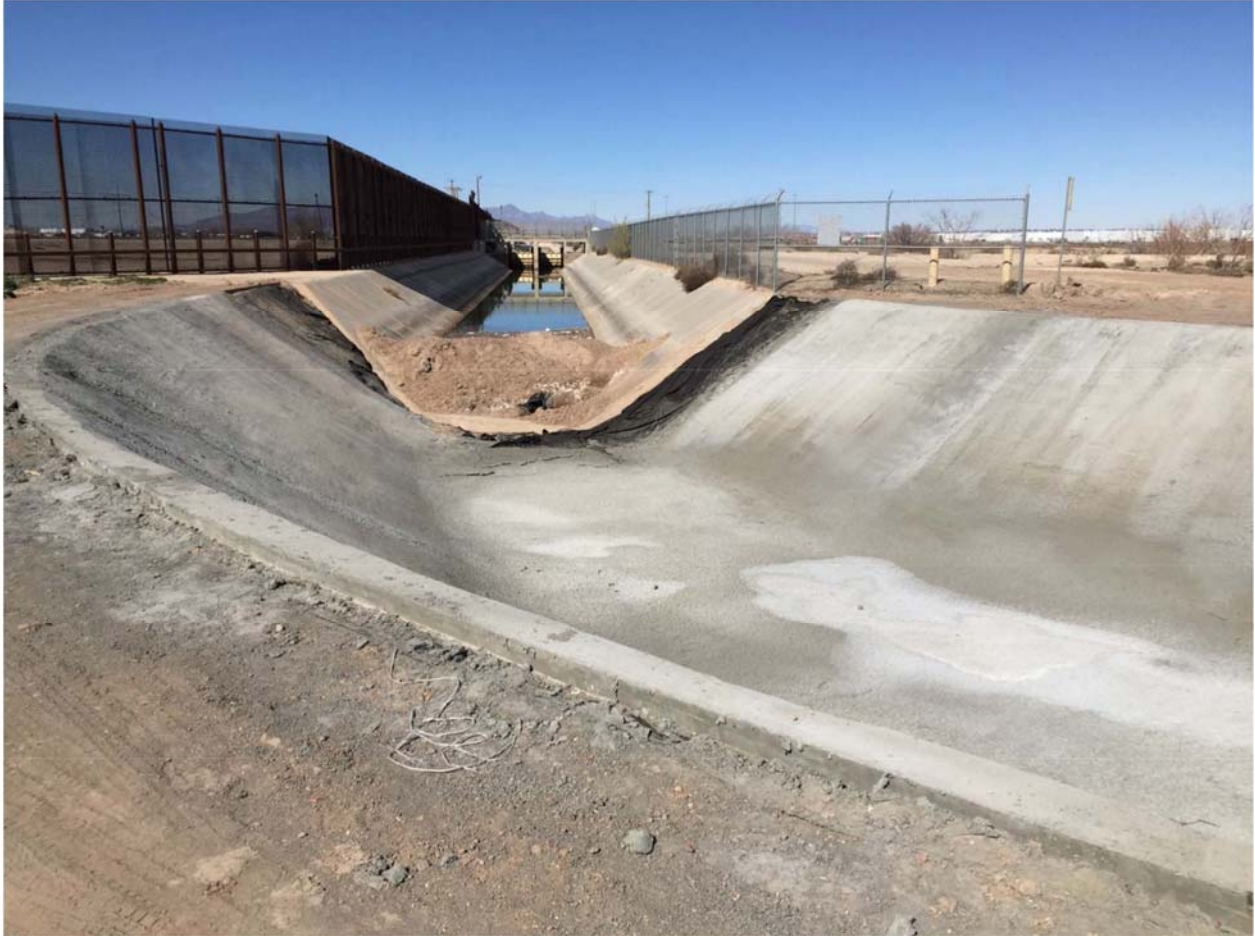
Location 1B. Dried shotcrete at the Riverside Canal heading. Additional lining needed at the transition from the American Canal. Photo dated 2/4/16.
