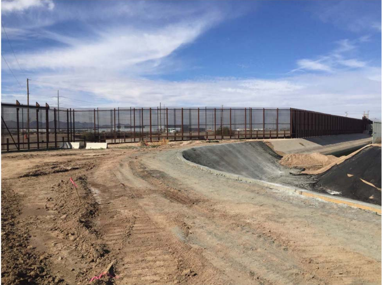
Location 1A. Shotcrete poured and dried on the right bank. Geofabric liner was placed on the left bank and canal bottom. Photo dated 1/15/16.
