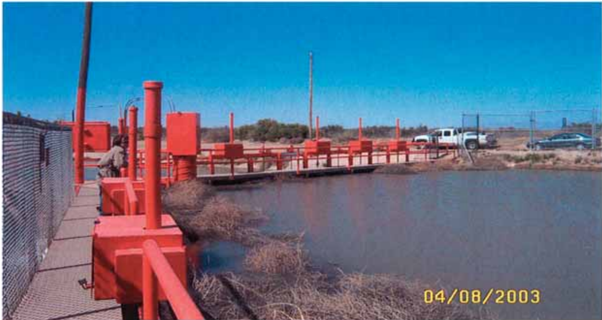
View of the upstream side of Franklin Check Structure (on the left) and the Partidor Check Structure (on the right).
