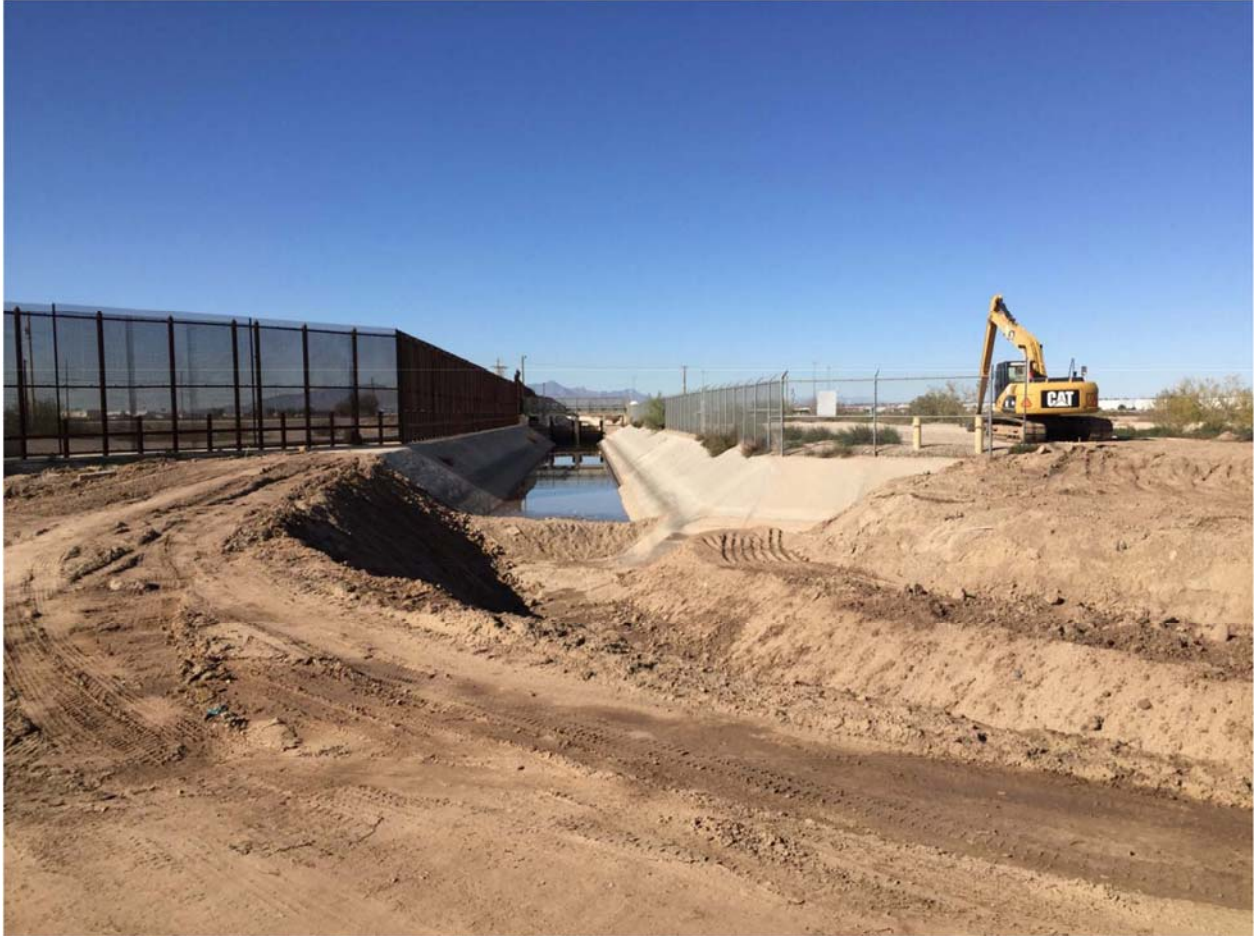
Location 1B. Additional earthwork and canal shaping at the Riverside heading. Photo dated 11/6/15.
