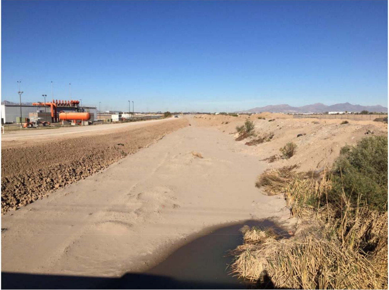
Location 6. Earthwork started on the right bank at Location 6. No work performed on the left bank yet. Photo dated 11/18/15.
