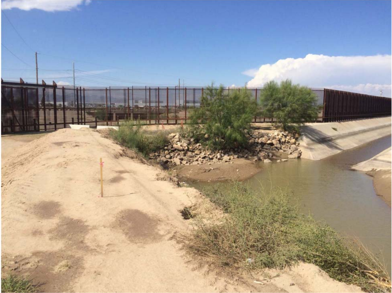
Location 1A. Pre-construction photo dated 10/21/15 of the Riverside Canal heading. The rock berm and small vegetation shown was removed as part of concrete lining work.
