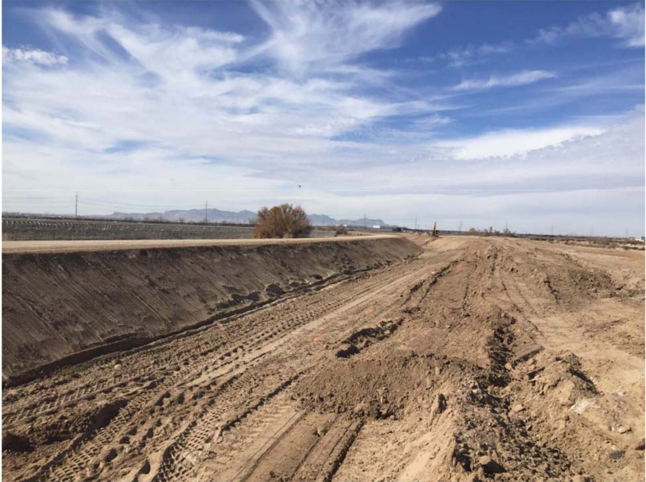
Location 5. Continued earthwork, vegetation cleared, and the piled dirt on the left bank was used to narrow the width of the canal cross-section. Photo dated 1/15/16.
