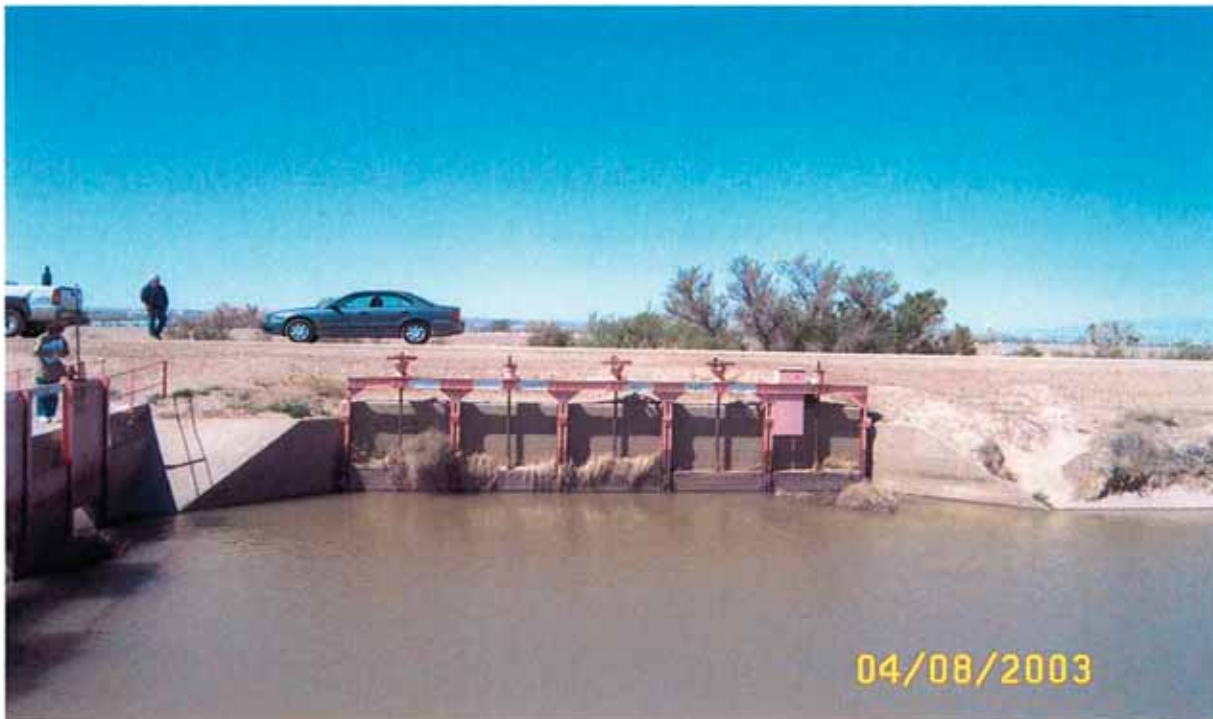
View of the existing Wasteway One and Check Structure on the left.
