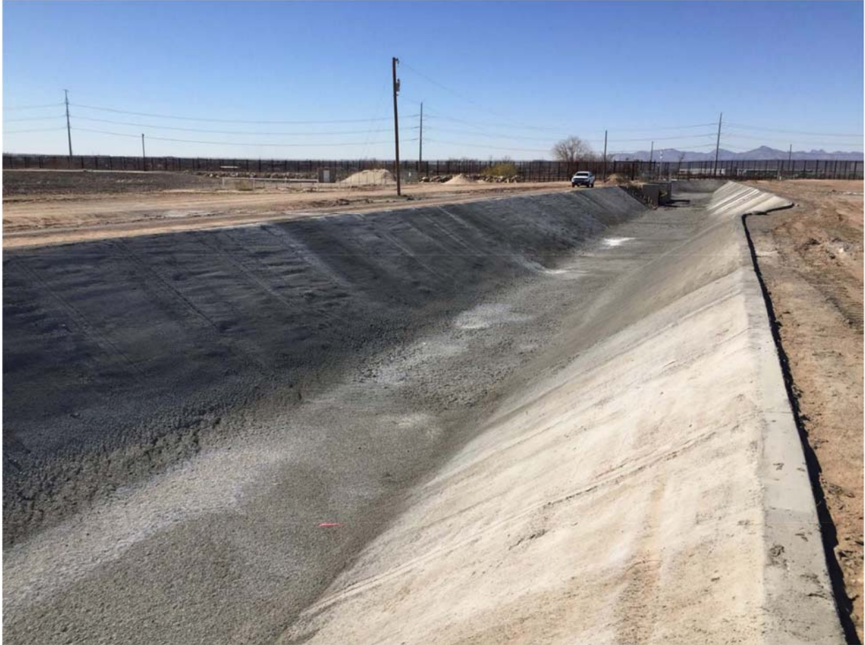
Location 4. Shotcrete in progress downstream from the intake structure for the JRWTP. Shotcrete used on the canal sides has dried. Canal bottom has not been smoothed. Photo dated 2/4/16.
