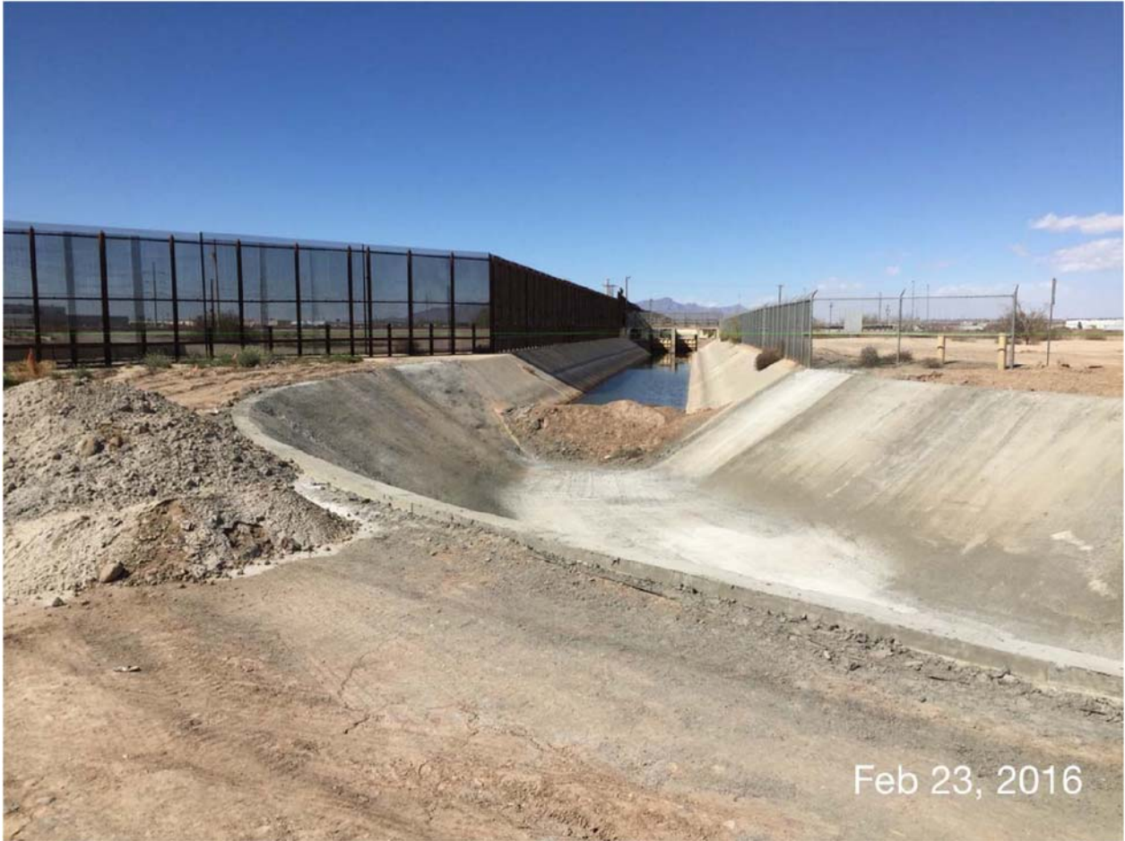
Location 1B. Transition from the American Canal to the Riverside Canal has been completed. The canal is fully lined. Photo dated 2/23/16.
