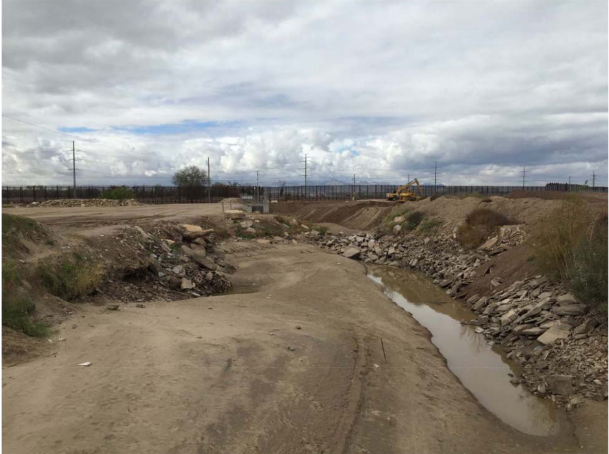
Location 3. Initial earthwork and cleanup at the intake structure for the JRWTP. The visible concrete slabs were disposed. Photo dated 10/30/15.
