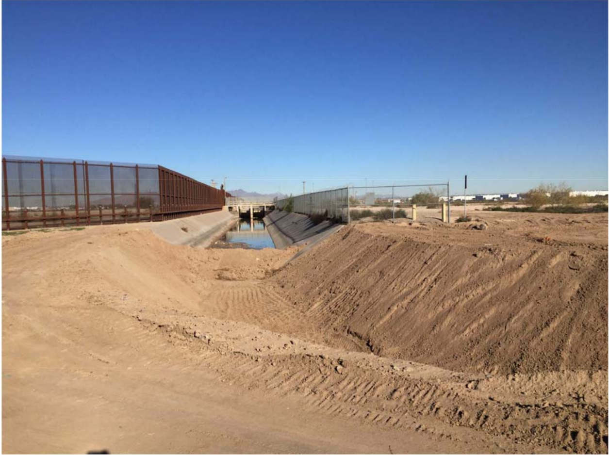
Location 1B. The earthen canal cross-section and transition from the American Canal was completed. Photo dated 11/18/15.
