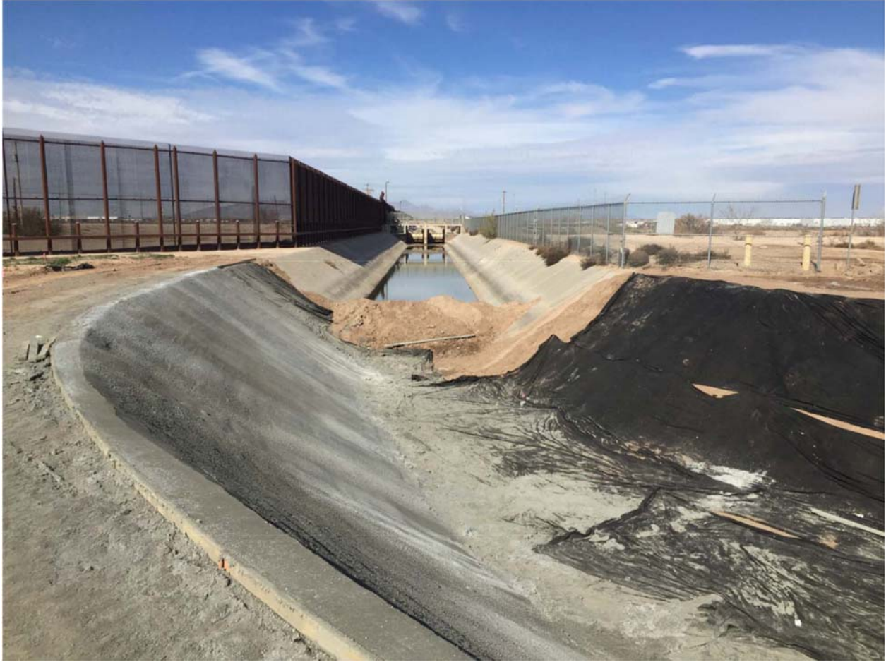
Location 1B. Shotcrete poured and dried on the right bank. Geofabric liner was placed on the left bank and canal bottom. Photo dated 1/15/16.
