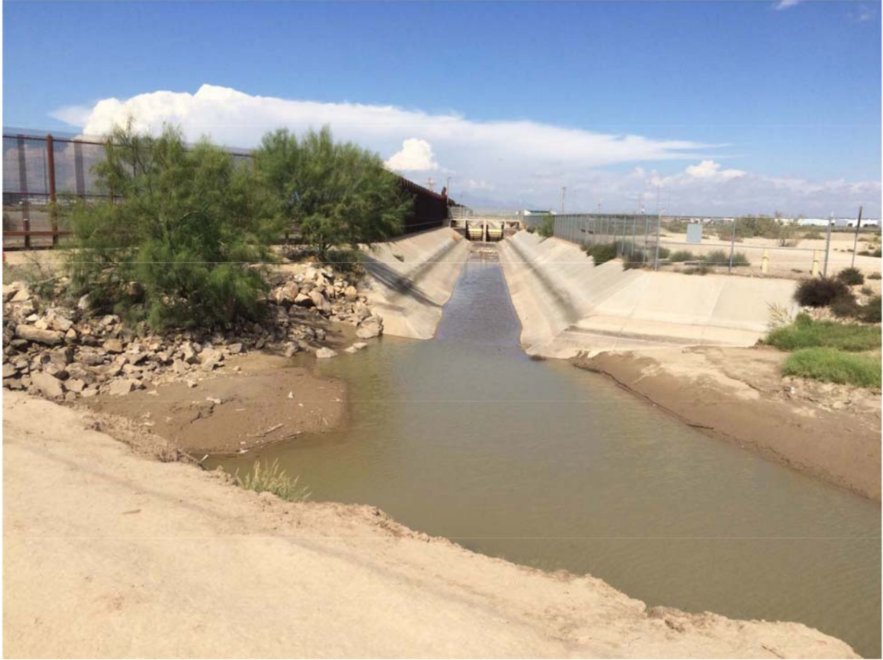
Location 1B. Pre-construction photo dated 10/21/15 of the Riverside Canal heading. Water flowing on the canal comes primarily from stormwater.
