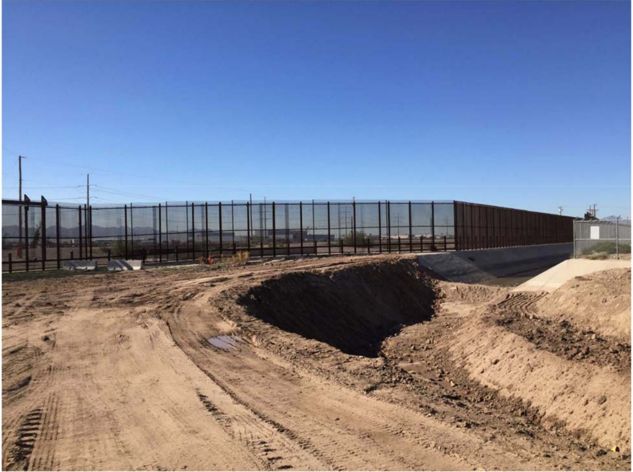
Location 1A. Additional earthwork and canal shaping at the Riverside heading. Photo dated 11/6/15.
