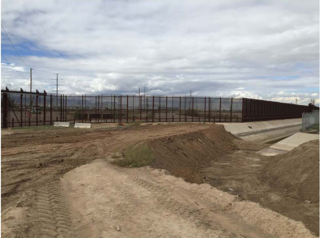
Location 1A. Initial earthwork at the Riverside Canal heading. The rock berm was removed and an earthen transition from the American Canal to the Riverside Canal was shaped. Photo dated 10/30/15.
