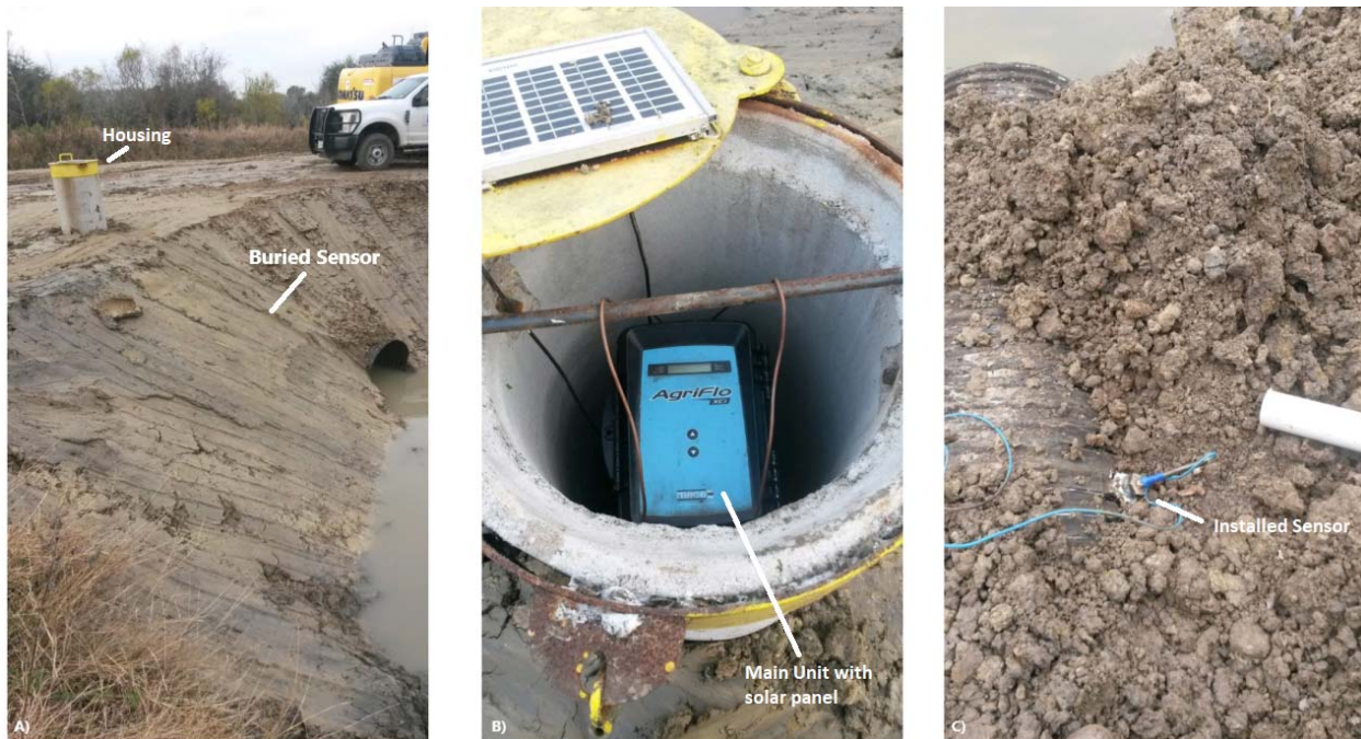
Figure 1-3 – Example Meter Installation - A) showing housing with easy access port, B) Agriflow meter installed within housing, with solar panel, C) on-pipe acoustic sensor transmits data via cable to the main unit.
