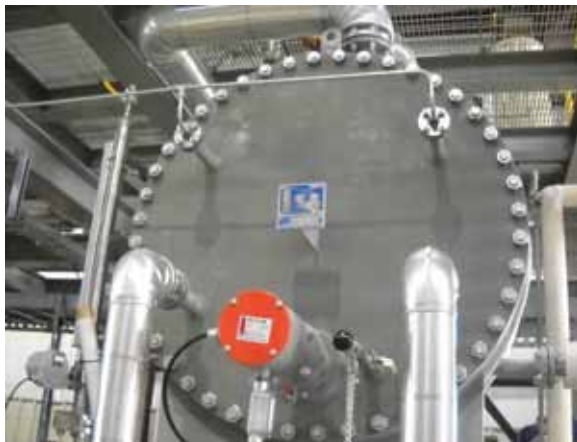
Assembled Evaporator (Front View)
