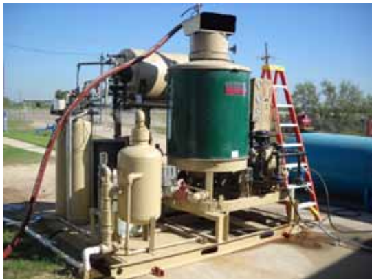
Figure 19. Fuel Oil Steam Plant for Start-up Testing
