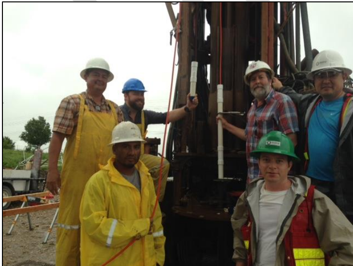
Photograph of the installation of the last Westbay casing piece in the multiport well. Photograph taken on 8/20/2016.
