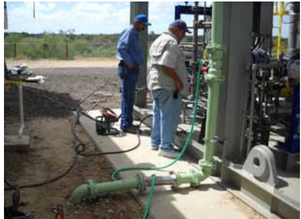
Figure 32. Well Water Input to the System
