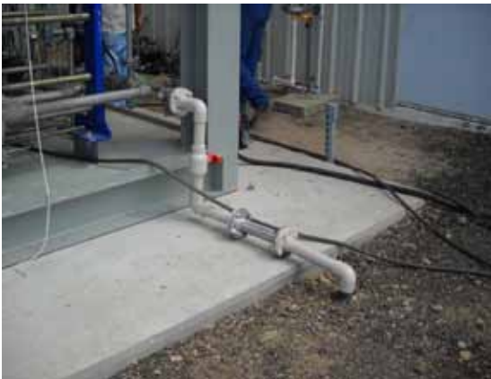
Figure 35. Brine Output Line to Brine Pit
