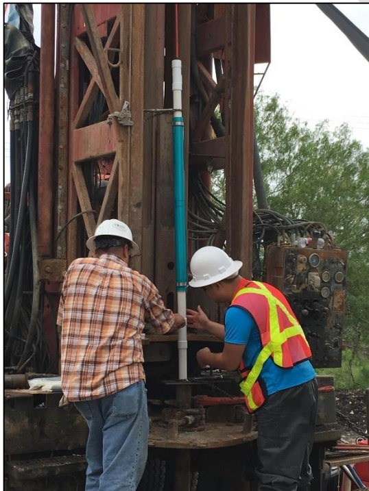
Figure 12. Photograph of assembly and testing of multiport coupling component. The coupling that connects the packer (blue, above) and the 10-ft casing section (white, below) is being pressure tested. Photo taken 8/20/2016.
