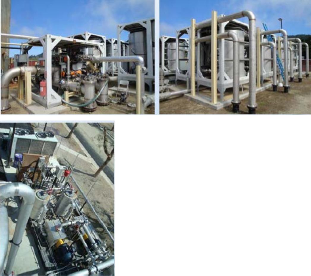
Figure 6.2 Gas Conditioning Skid
