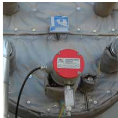
Figure 20. Start-up and Supplemental Heater in an Evaporator
