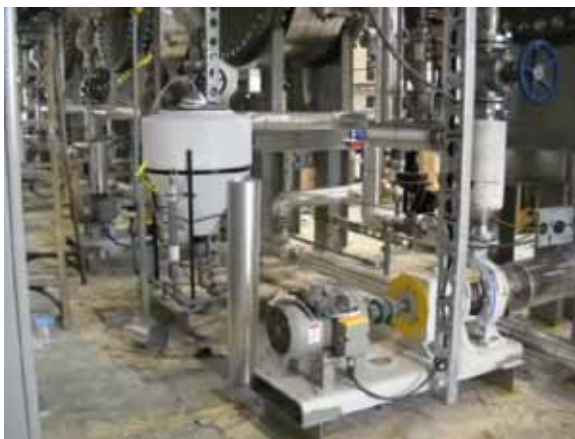
Figure 15. Brine Recirculation Pumps and Chemical Treatment Tank
