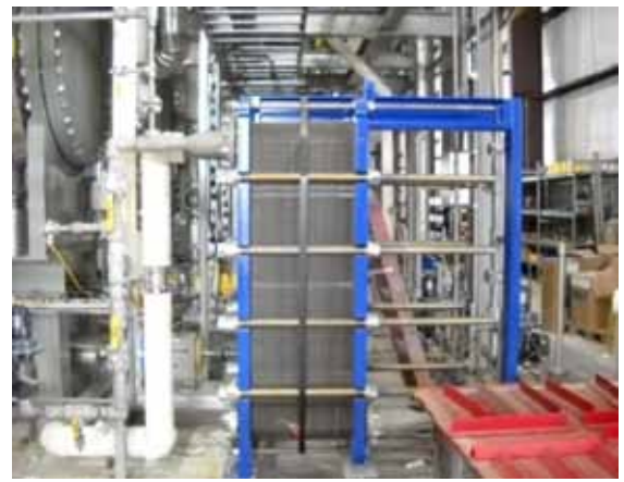
Figure 14. Sensible Heat Exchanger to Preheat Incoming Raw Water
