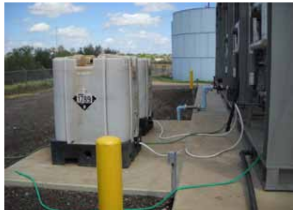
Figure 36. Chemical Tanks for Pre-Treatment of Well Water
