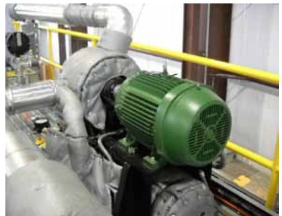
Figure 16. Star Rotor Compressor Installed on Top Platform
