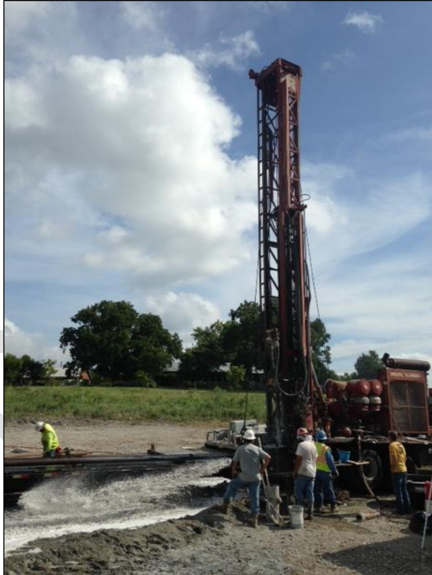
Figure 5. Drilling and development of the borehole for the multiport monitor well. Photo taken on 8/11/2016.
