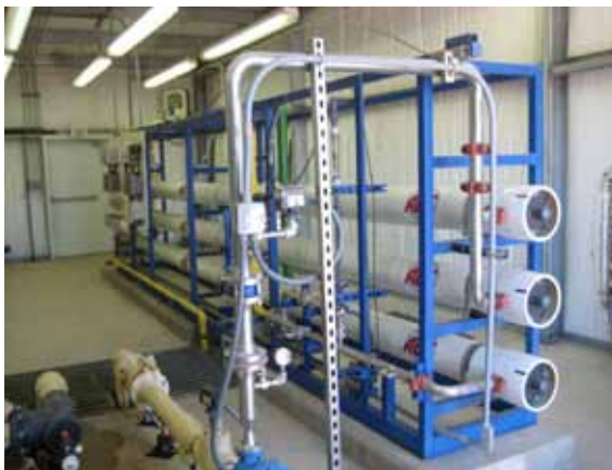
Figure 25. RO Plant Membrane Rack
