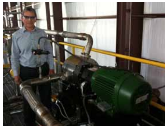
StarRotor Compressor Installed
