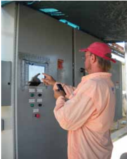
Figure 17. Pilot Plant Control Panel
