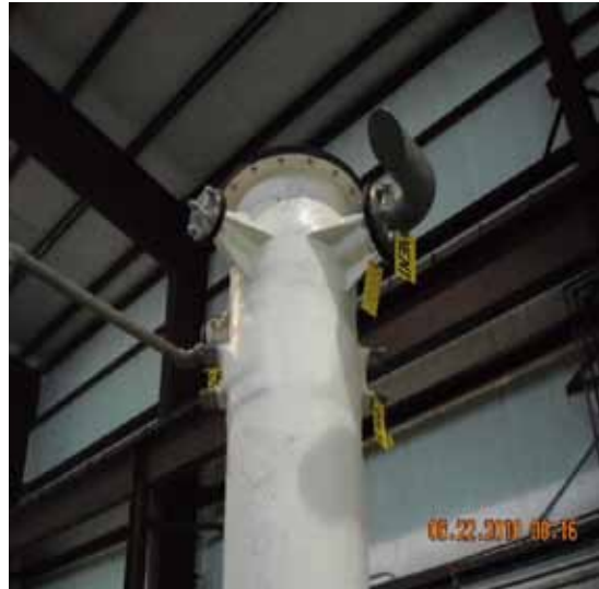
Figure 18. Carbon Dioxide Scrubber
