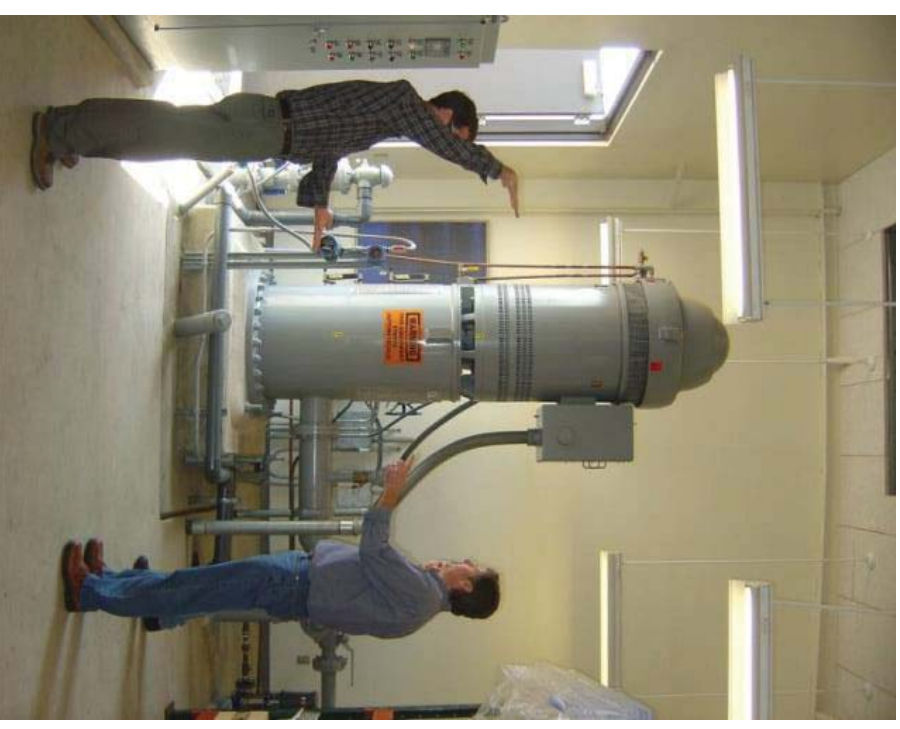
Calleguas MWD, California
