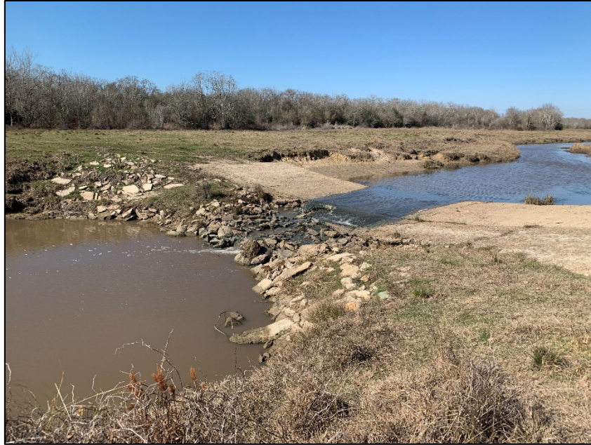
Figure 17. Barrier to flow on Big Boggy Creek. This structure (barrier 1 in Table 2 & Figure 16) does not appear to have culverts and instead allows the water to flow over the top.
