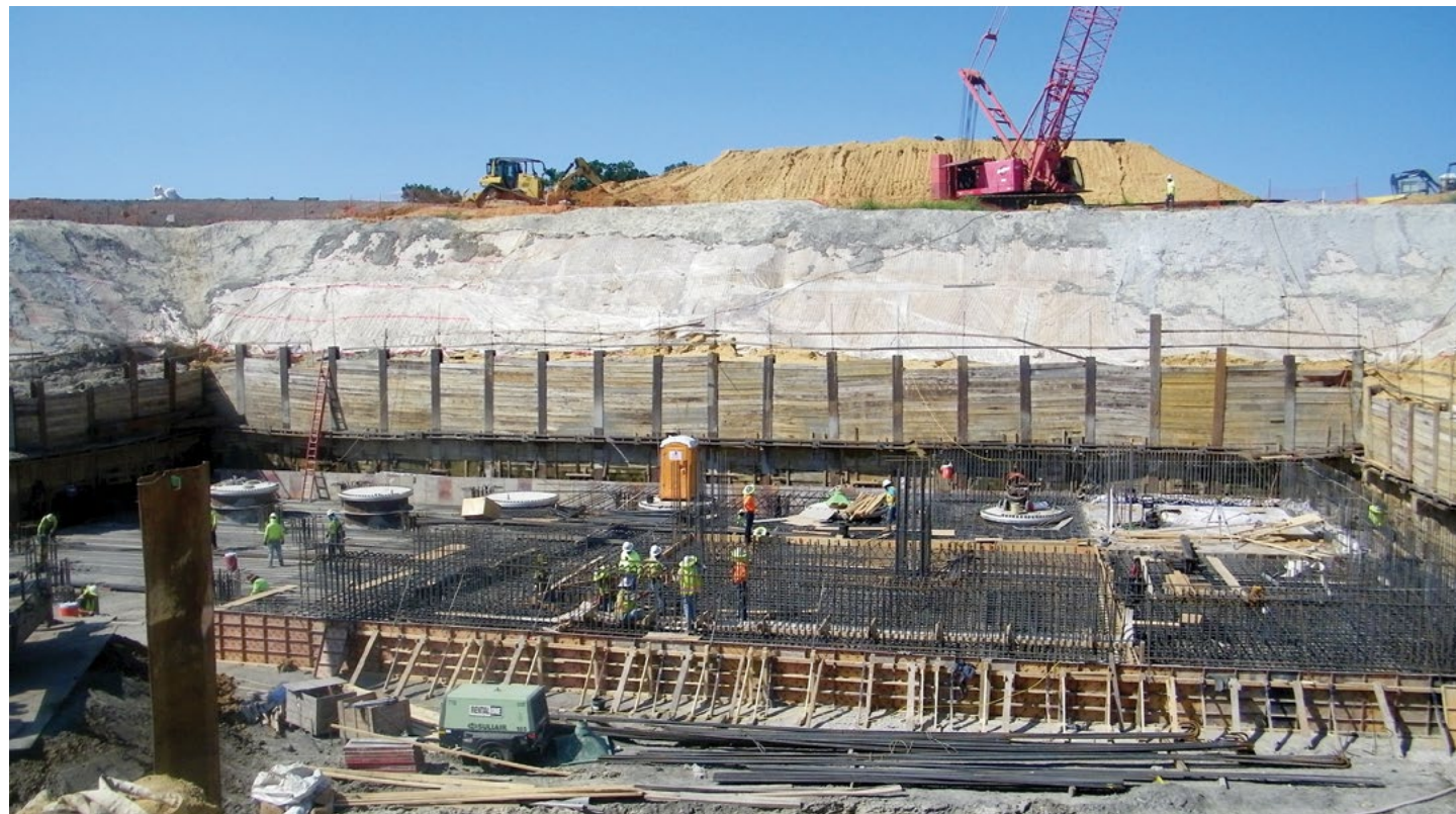
Tarrant Regional Water District and Dallas Water Utilities have partnered to finance, plan, design, construct and operate the Integrated Pipeline Project and have benefitted from cost savings through SWIFT.
