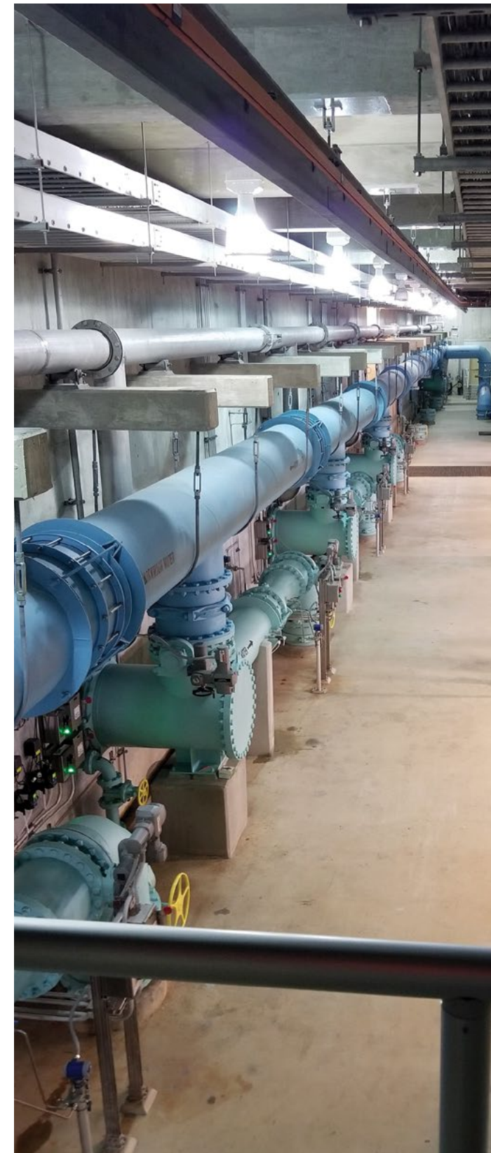
Brushy Creek Regional Utility Authority is using SWIFT financing to develop additional water supplies for its customers. Photo courtesy of BCRUA.
